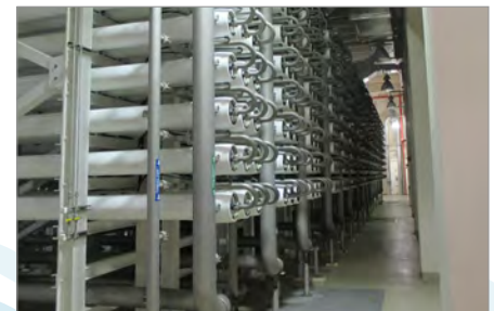
Figure 5: Larger RO Facility Example
