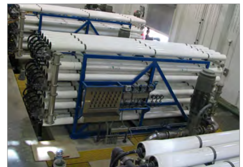
Figure 2: A Plant With Multiple RO Skids
