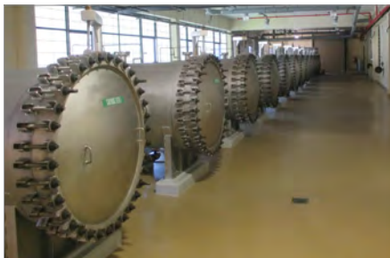
Figure 3: Cartridge Filter Housings for Pretreatment
