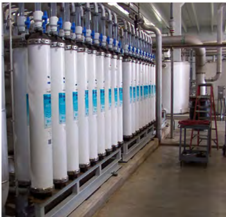
Figure 2: Example of skid mounted UF modules
